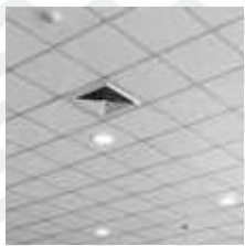
CEILING GRID FALSE CEILING
